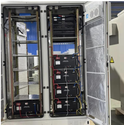
Advanced Solar Power System in South Africa ...
