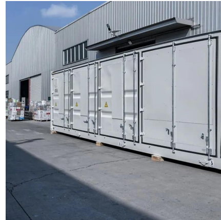
Battery container for electric car batteries . RETRON 4000 // ...
